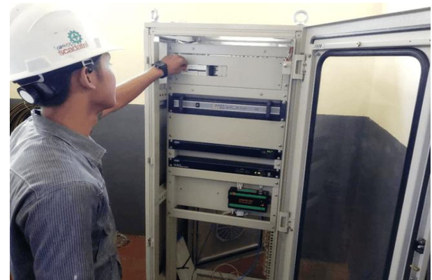
Figure 11. GH Manembo Inverter Device
