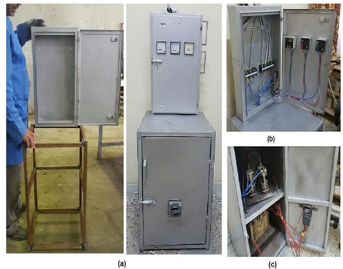
Figure 13 the transformer/rectifier panel
