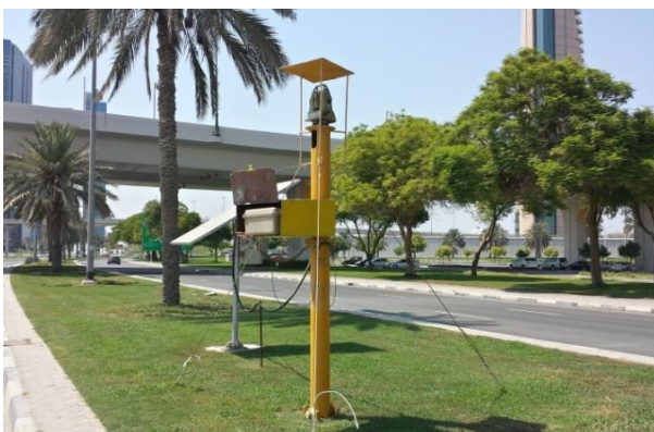
Figure 2: Installed ATS on site with control box and solar panel power supply
