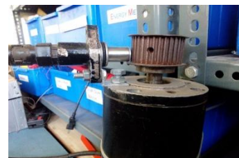
Figure-3: Connection to the motor and the speed sensor
