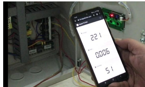
Fig 8: Testing of the PLTMH Control System via Smart Phone
