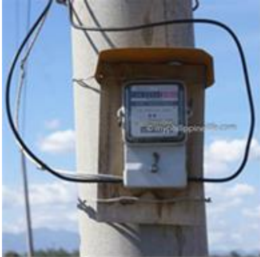
Fig 2: Pole-mounted smart prepaid meter
