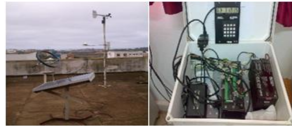
Fig 1: Meteorological station with the data logger Campbell CR10X
